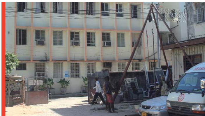
Soil testing for the new clinic on the parking lot next to the Shree Hindu Mandal Hospital
